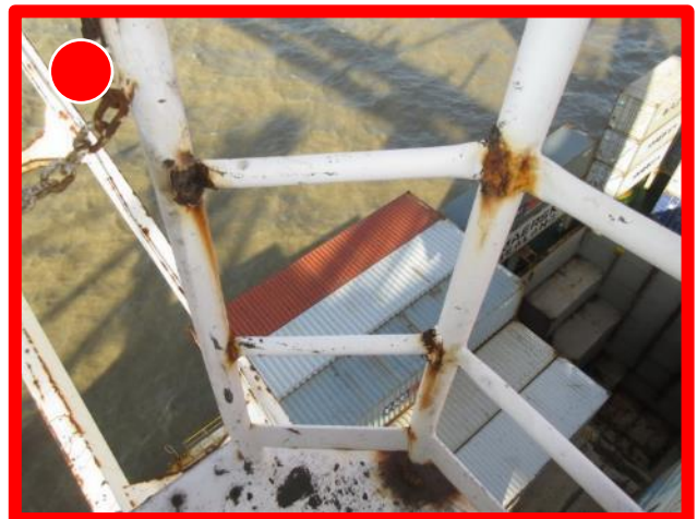
Excessive corrosion on topside handrail
