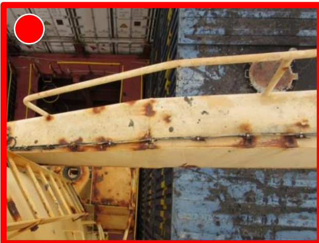
Jib with spots of excessive corrosion
