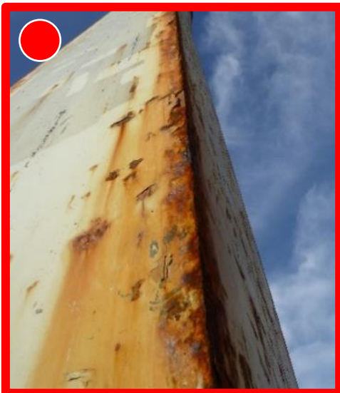
Excessive corrosion along pedestal edge
