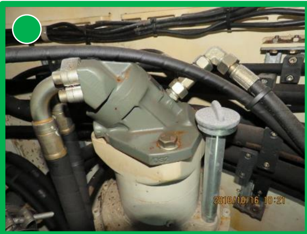
Superficial corrosion on valve block
