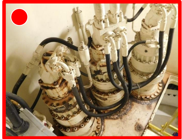
Slewing motors with excessive corrosion
