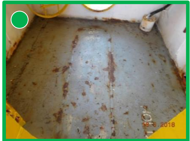
Progressing corrosion on entrance deck
