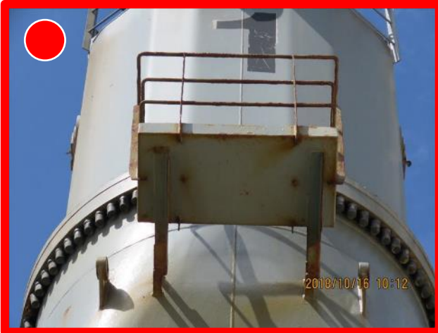
Excessive corrosion on external platform supports and railing
