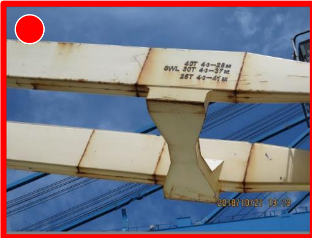
Jib with (localised) excessive corrosion
