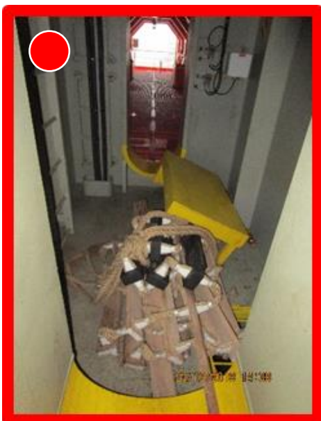
Objects in pedestal structure obstructing passage
