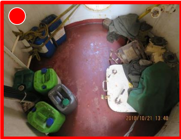
Pedestal entrance with objects obstructing passage
