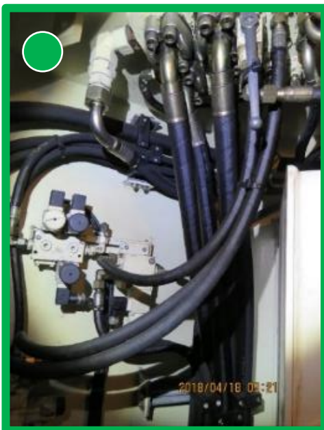
Hoses sound, shiny appearance not related to leakage because there is no dripping of oil
