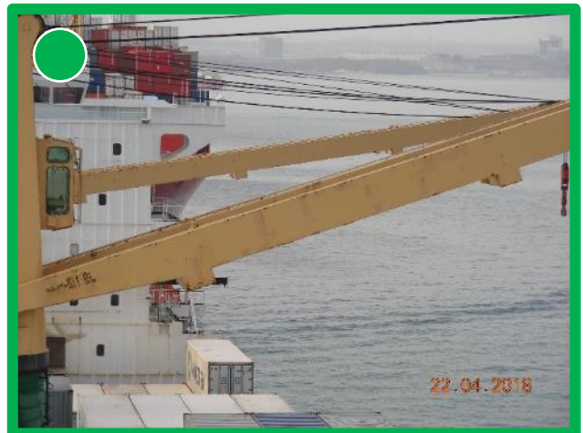
Progressing corrosion on jib
