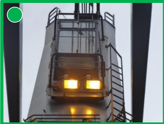
Operator's cabin with superficial corrosion
