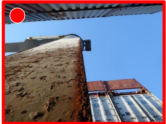
Excessive corrosion along pedestal
