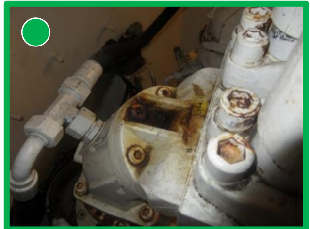
Progressive corrosion on valve block
