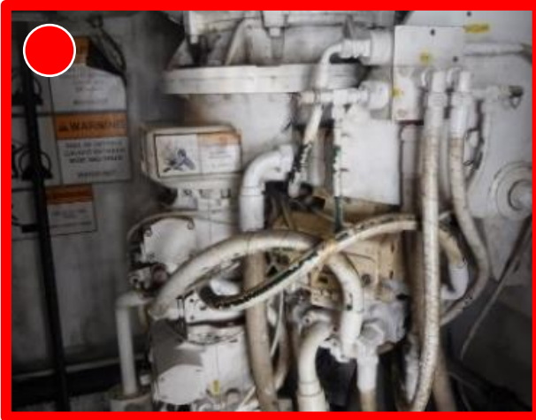
Hydraulic hoses stained and with paint
