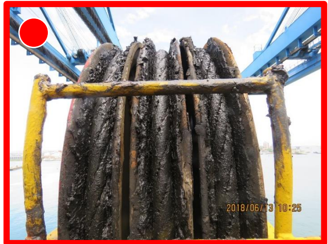
Wire sheave with corroded edges
