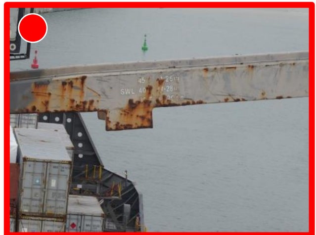
Excessive corrosion along jib
