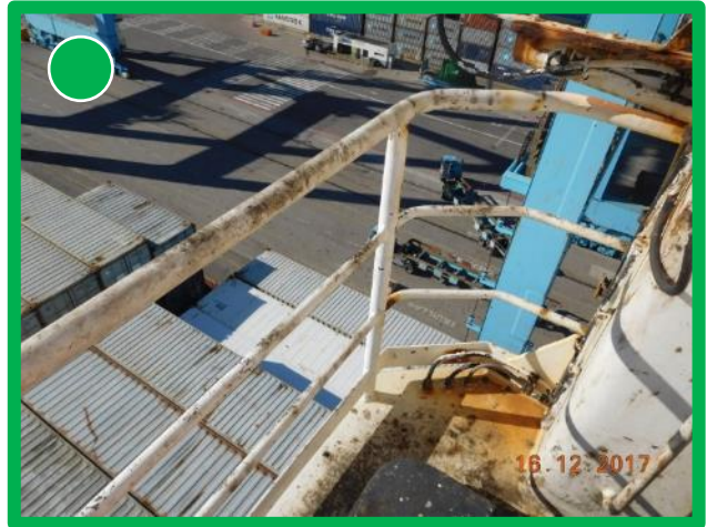
Handrailing with superficial corrosion
