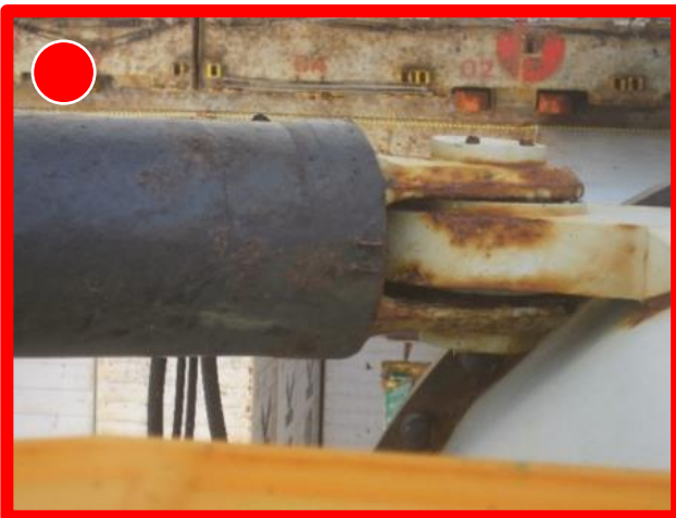
Luffing cylinder mounting with excessive corrosion
