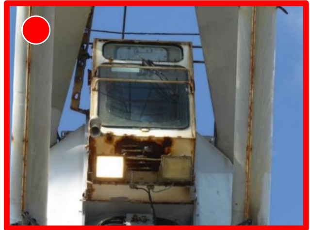
Operator's cabin exterior with excessive corrosion (and one inoperative flood light)
