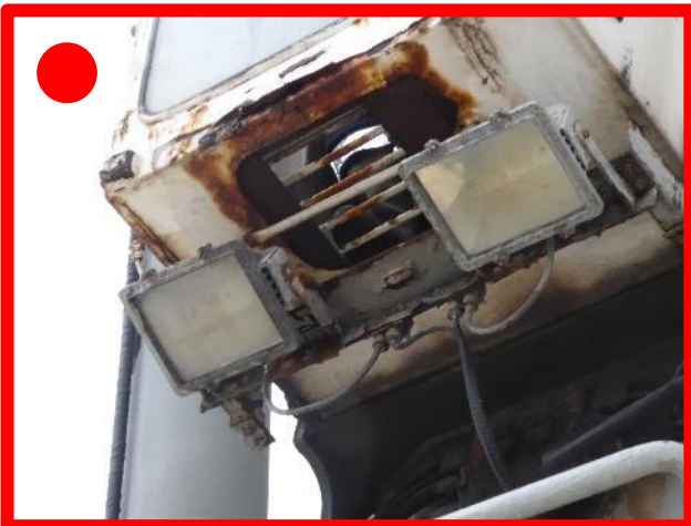
Cabin structure excessively corroded / local wastage
