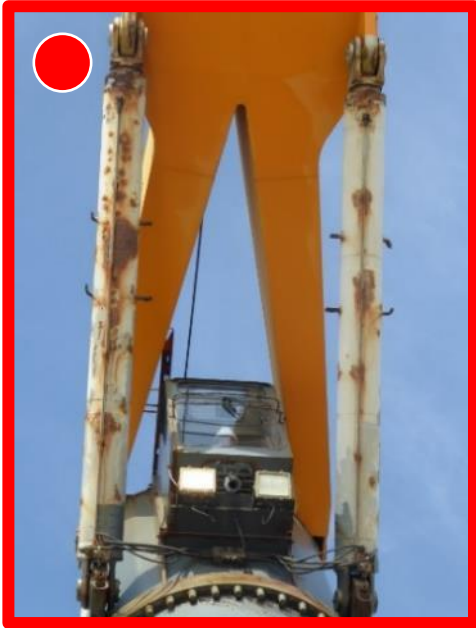
Luffing cylinders with excessive corrosion
