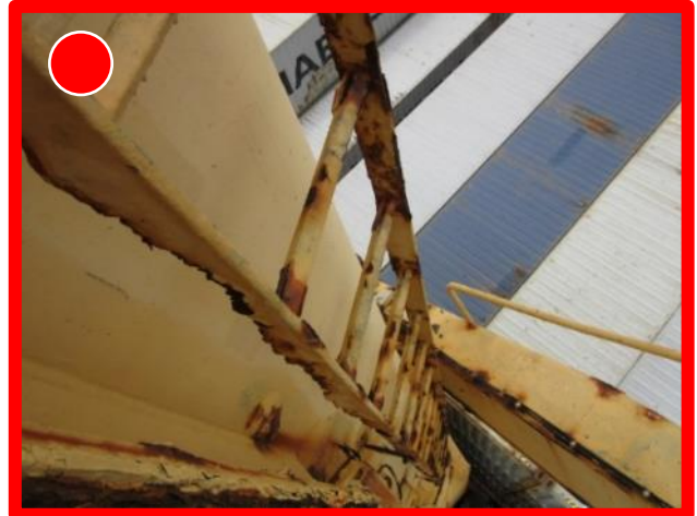
Excessive corrosion / wastage on pedestal ladder
