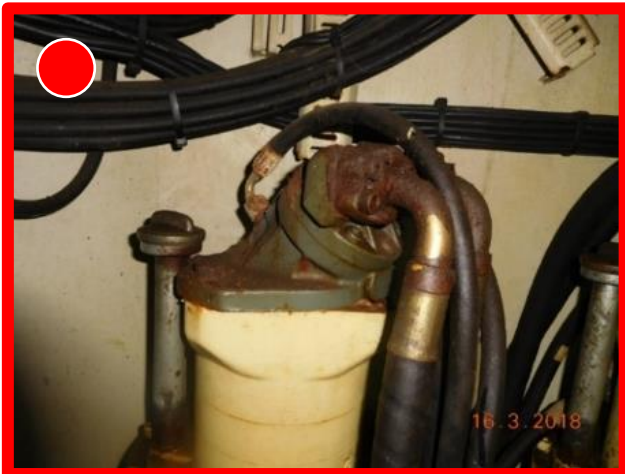
Excessive corrosion on valve block
