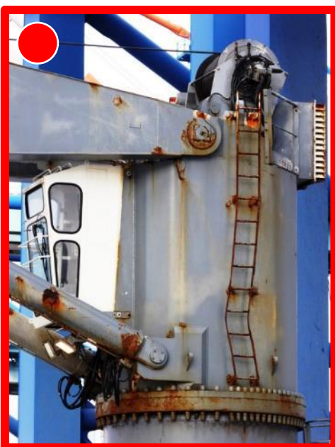
External ladder with excessive corrosion and distorted.
