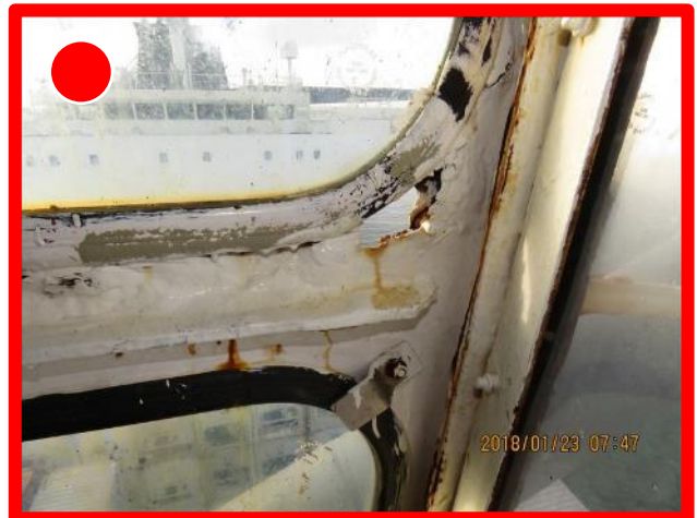
Inside view: cabin structure wasted
