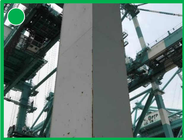
Superficial corrosion along pedestal edge
