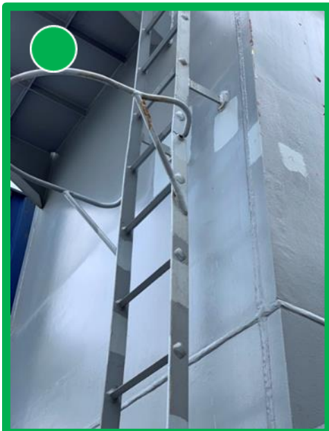
Minorly damaged/deformed ladder safety ring
