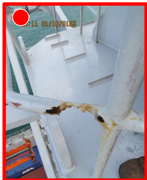
Topside handrailing with wastage
