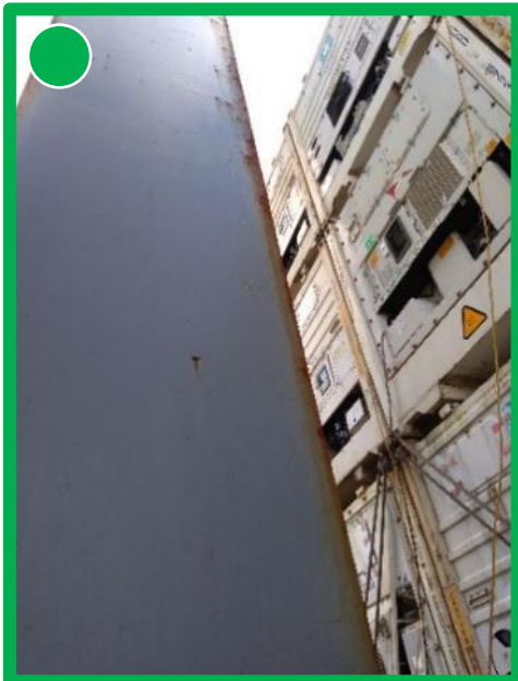
Superficial corrosion along pedestal edge
