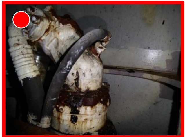
Excessive corrosion on valve block
