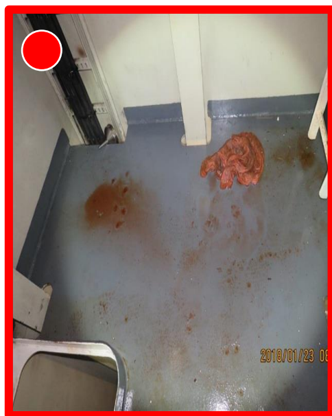
Intermediate crane platform, oily and slippery
