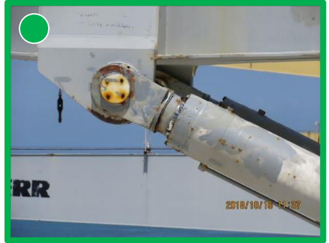
Limited corrosion on jib / luffing cylinder mounting
