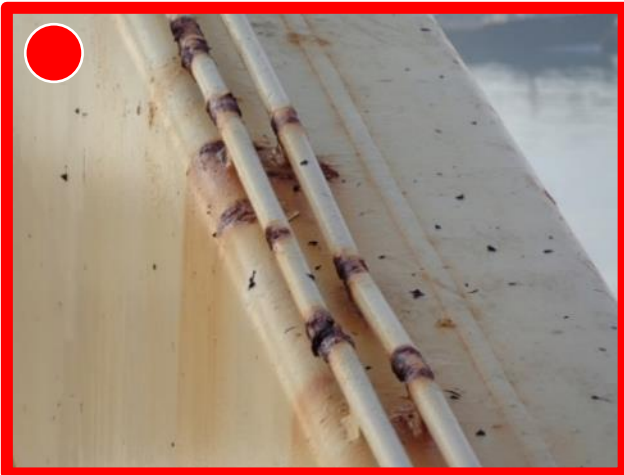
Excessive corroded cable protection piping
