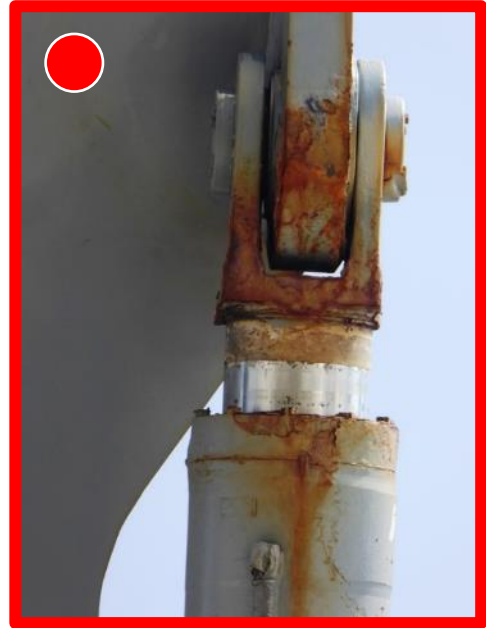
Excessive corrosion on jib mounting
