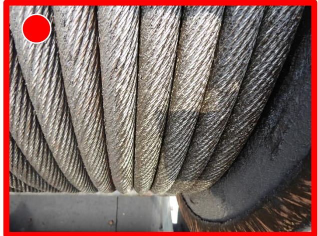
Wire dry, lacking grease
