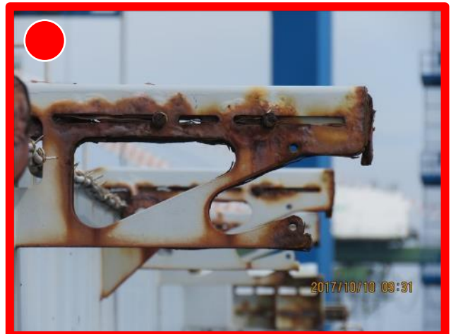
Excessive corroded grating support
