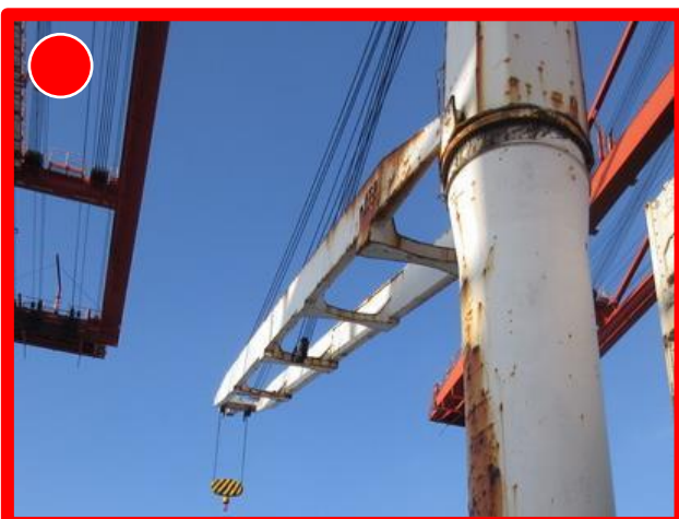
Jib with excessive corrosion (also on pedestal and slewing ring)
