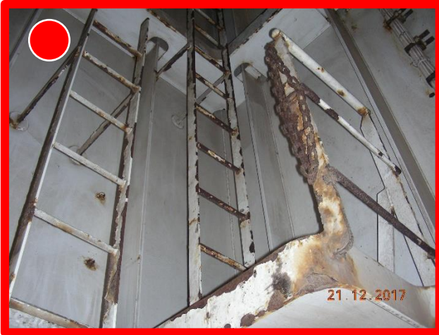
Interior and ladders with excessive corrosion
