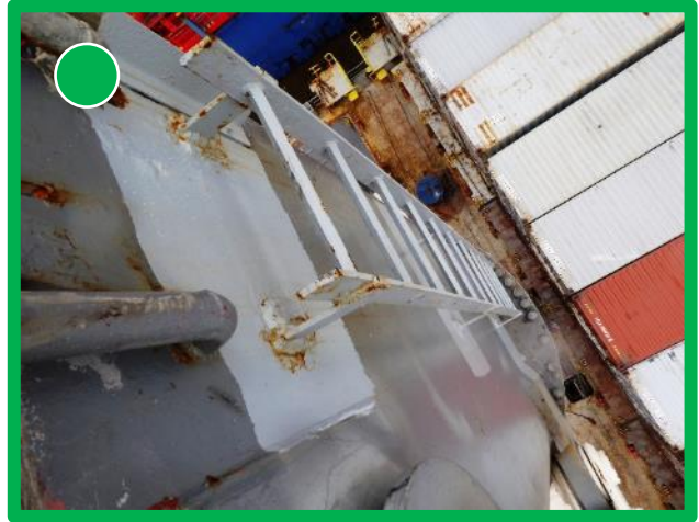
Ladder with some progressing rust
