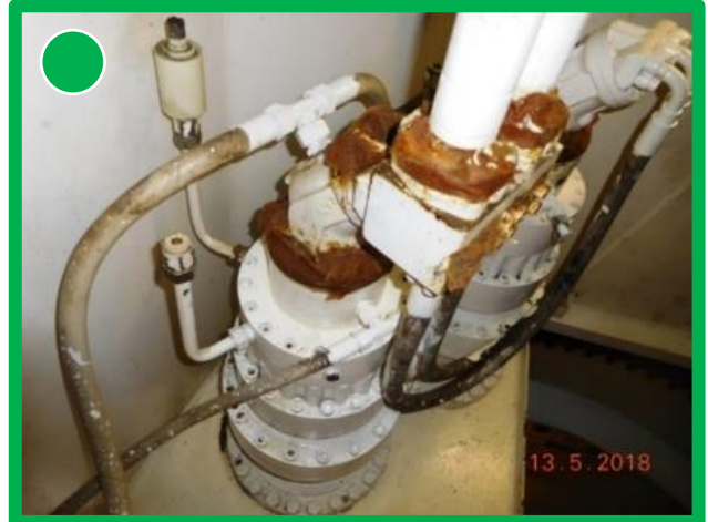
Anti-corrosion tape on slewing motor couplings
