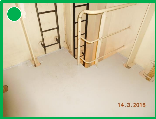
Crane interior, clean and safe
