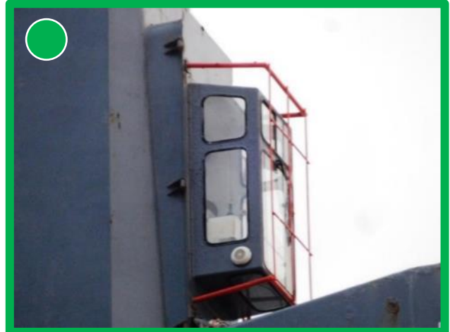
Operator's cabin with superficial corrosion
