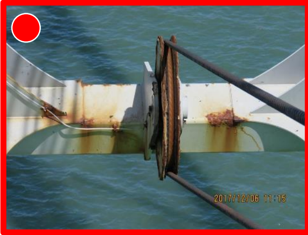
Jib with local excessive corrosion
