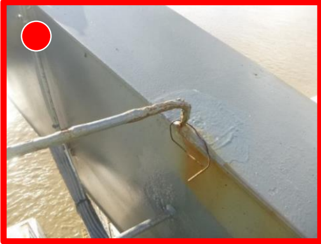
Excessive corrosion on handrail at the base of the jib
