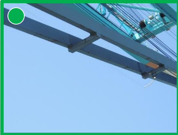
Superficial corrosion on jib
