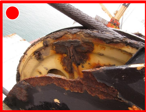
Wire sheave with excessive corrosion
