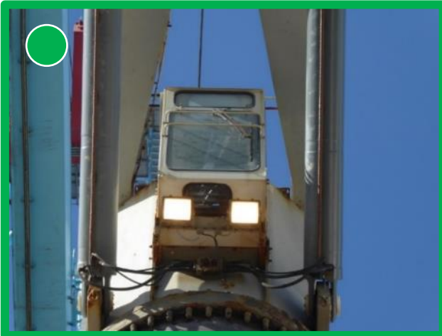
Operator's cabin with superficial corrosion
